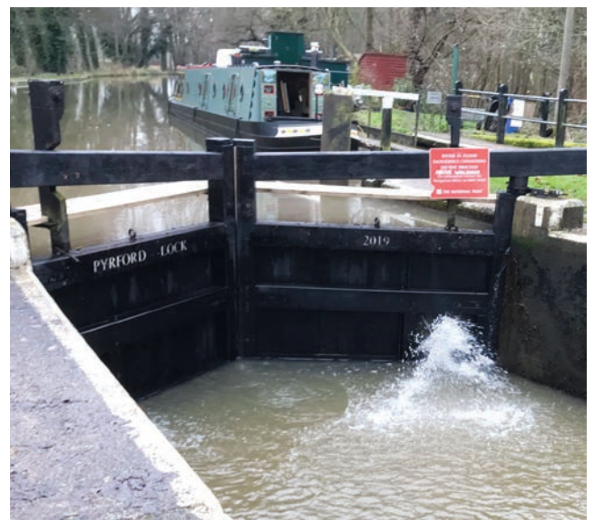
Even new lock gates never seem to be completely watertight
