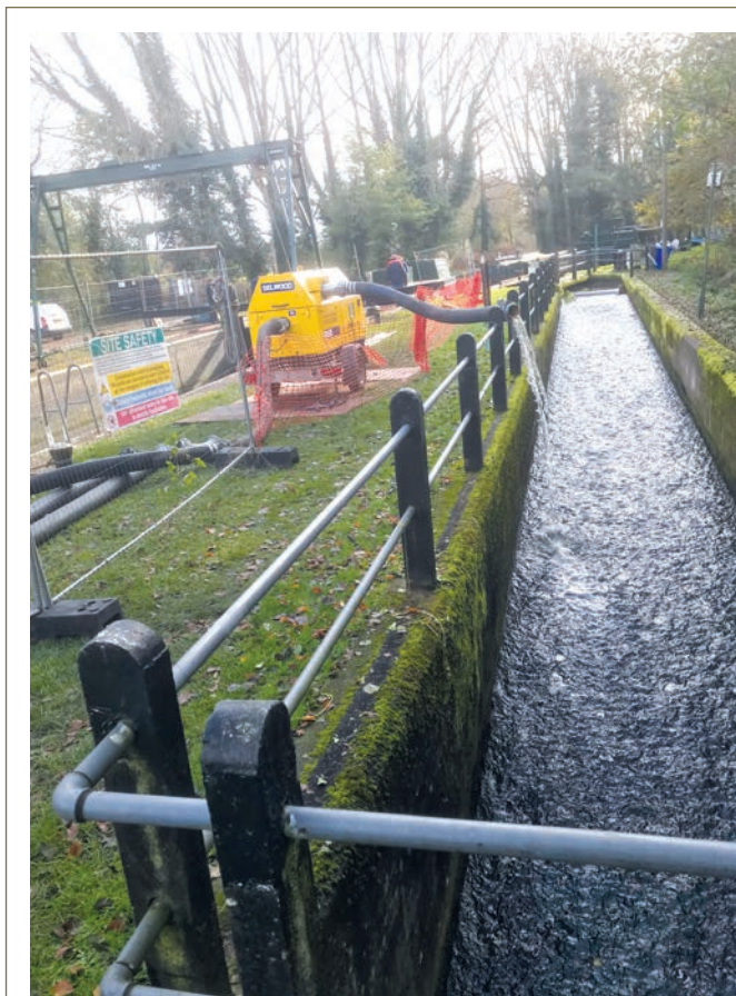
Water is pumped from the lock into the bypass channel
